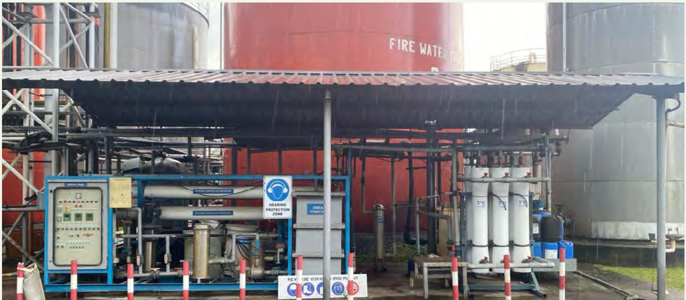
Our water management includes treating wastewater for general use.
